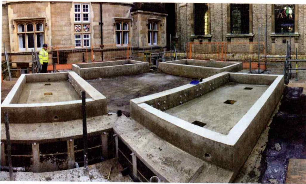
Left: Severely restricted access to the 17x22 metre site meant that the only piece of powered machinery available was a mini digger. The rest of the work relied on manual labour.
